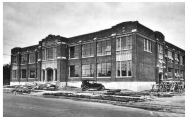
Morton M. McCarver Intermediate School (previously McCarver Elementary) by Hill & Mock architects, shown under construction in 1925. Photo courtesy of Tacoma Public Library.
