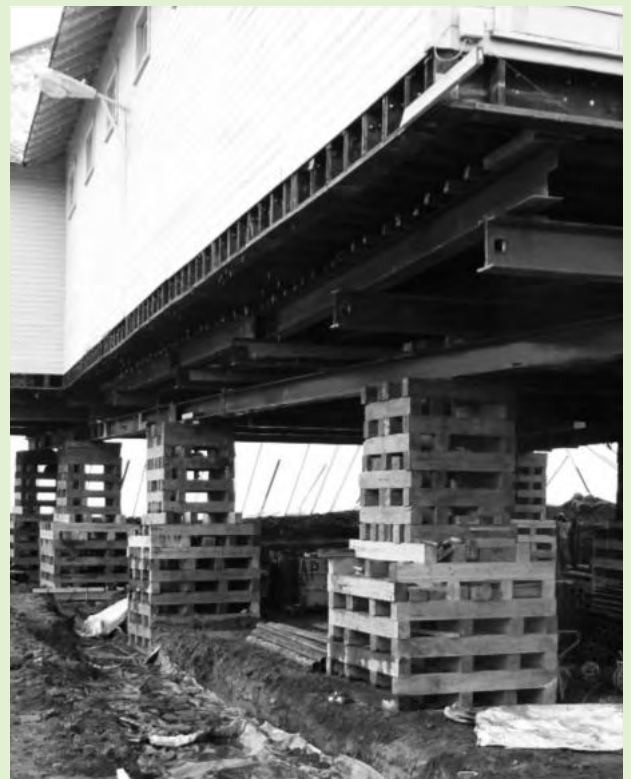
Roslyn's Old City Hall under construction. Photo courtesy of BOLA Architecture + Planning.
