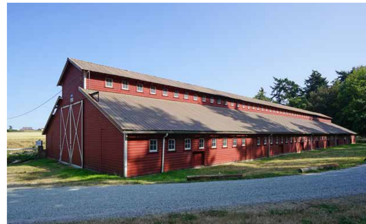
Above: View of the Sherman Hog Barn from Hill Road before rehabilitation in 2007.
