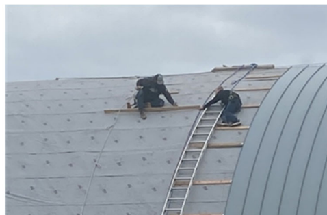
Progress Report. This photo clearly shows the work underway, making it an informative photo for grant administrators. (Vekved Barn, Whatcom County)
