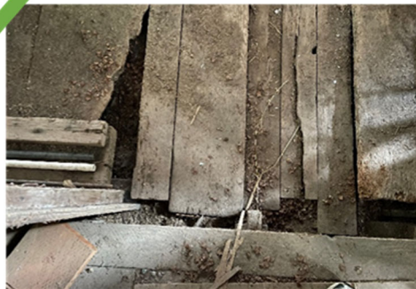
This photo shows clearly the damaged floor in its larger context. (Wild Isle Farm, King County)
