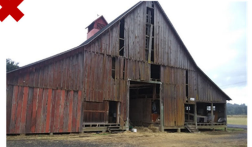
The left corner and peak of roof are cut off in this photo. (Gregory Farms, Lewis County)
