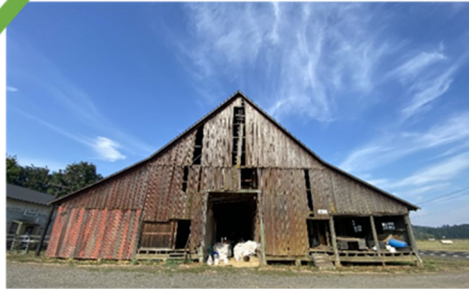
The corner and roof shape are clearly visible in this photo. (Gregory Farms, Lewis County)
