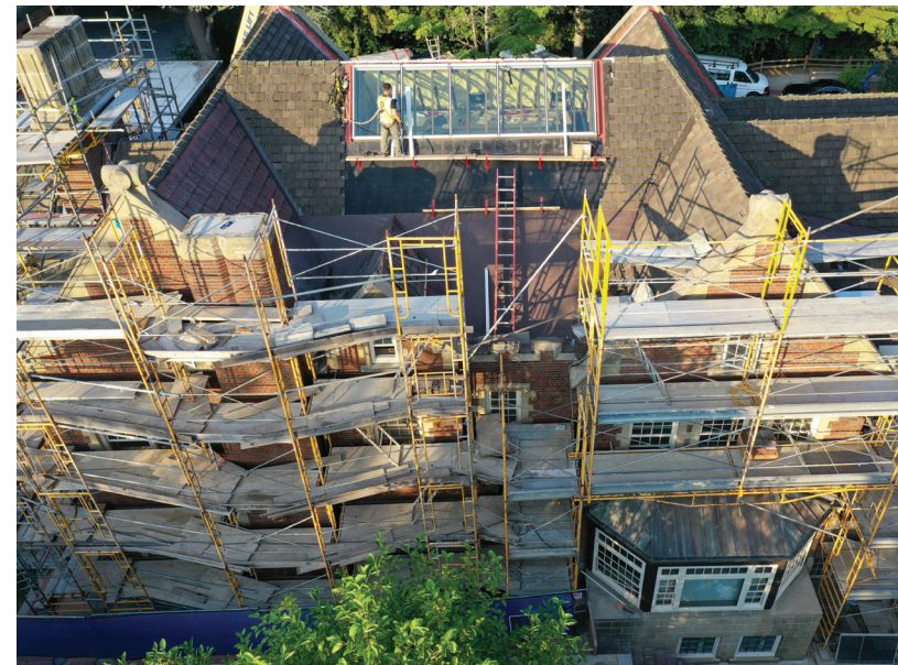
Left: Glass is installed in the building's new skylight atrium, while scaffolding enables masonry restoration and other projects around the exterior.
